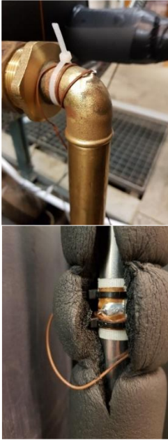
Figure 4: Thermocouples immersion sleeves: surface and elbow thermocouples
