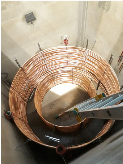
Figure 1 : Two heliocidal heat exchangers in a rainwater tank - Location : Saverne, France.
