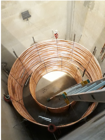
Figure 1 : Two helicoidal heat exchangers in a rainwater tank - Location : Saverne, France.
